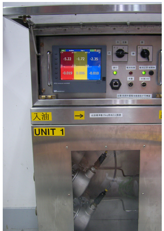
Overview of oil flow monitor
