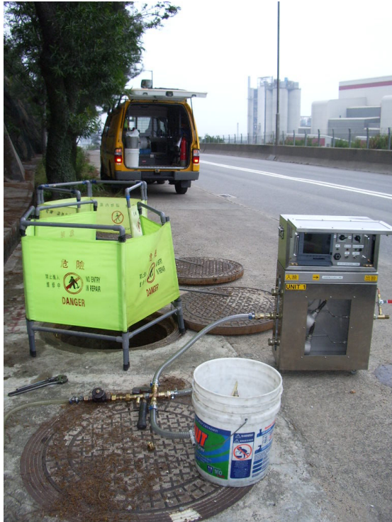
On site monitoring of cable oil leakage
